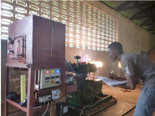
During training, a Biomass Brother runs tests and records data on the 5kW Lister Engine running on crude palm oil (CPO)
