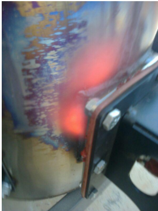
An example of localized overheating due to an internal fire caused by an air leak from a poorly re-sealed interface.
